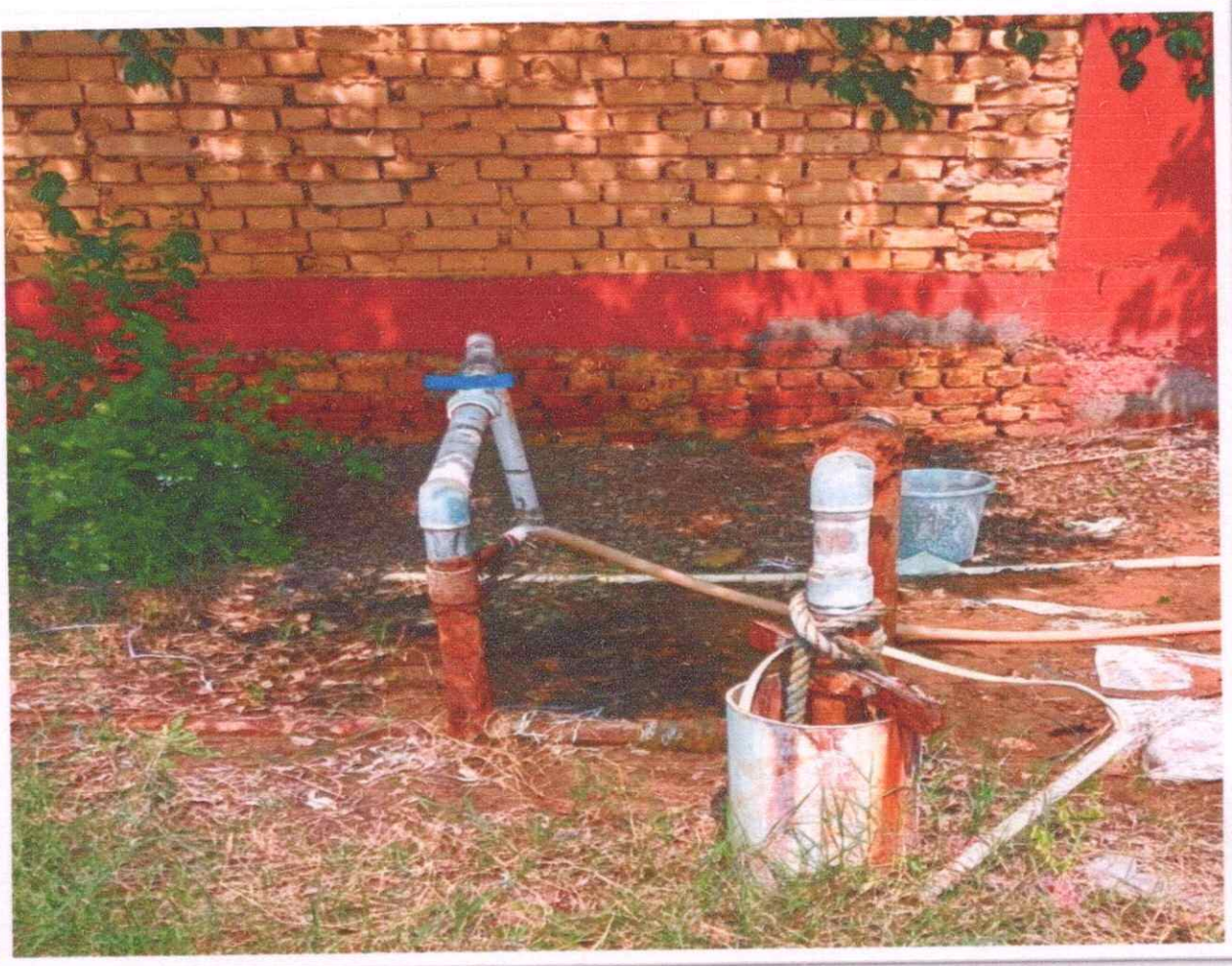
Recharge Bore well-001
