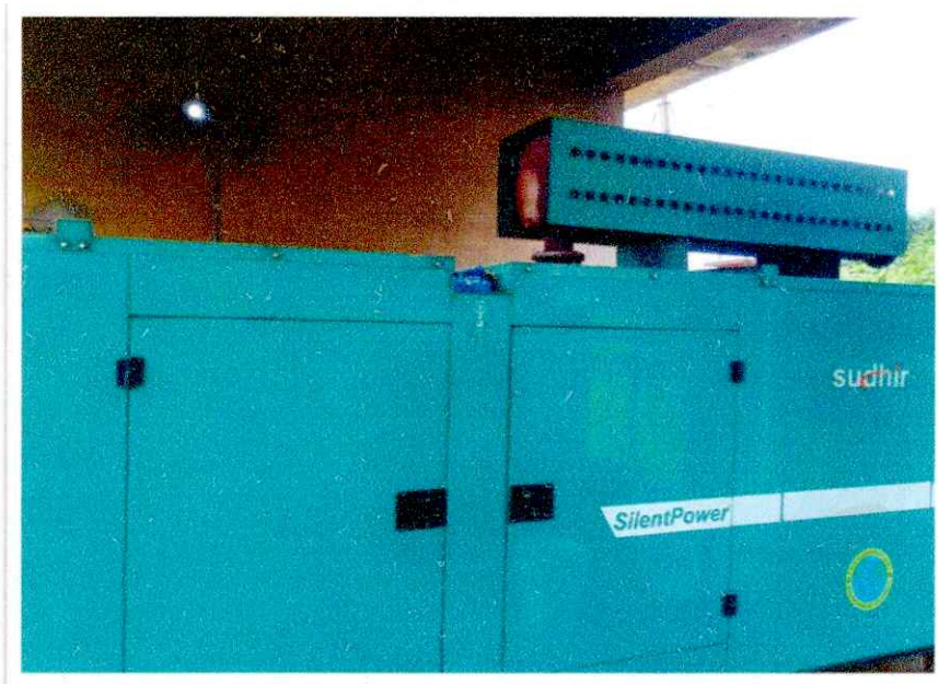
Diesel Generators Inside the Campus
